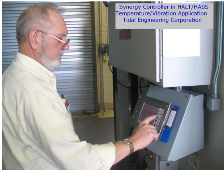
Figure 1, Synergy Controller Installation
